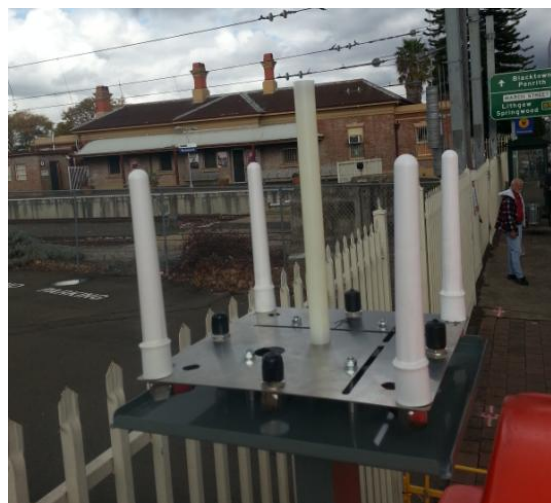
Magenta cube removed showing 4 Omni Directional Antenna
