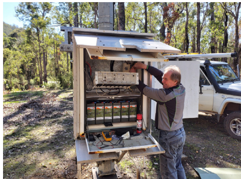
Telstra employee Garry Schreiber restoring lines for a school camp near Dwellingup, WA.
