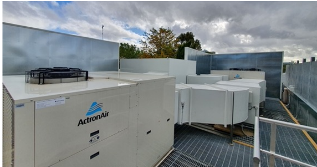
New roof top air conditioning plant
