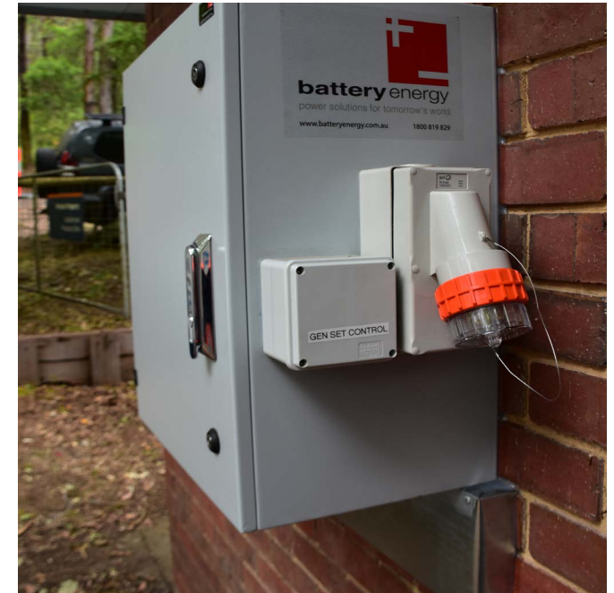
Automatic transfer unit located at Powelltown Exchange
