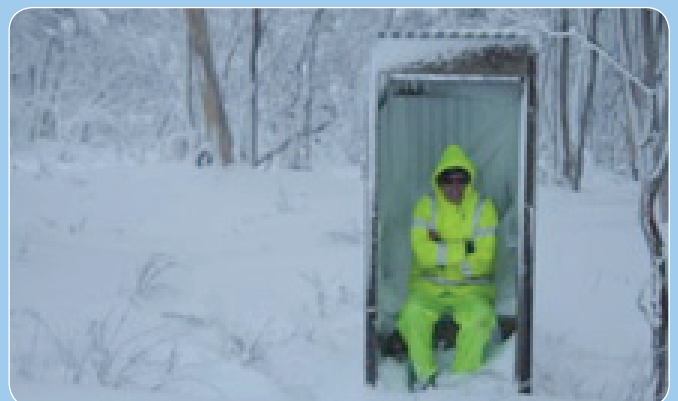
Top: The completed Mt Matlock installation features 7.5m high poles with solar tilt poles, which can be lowered for installation and maintenance, and are tilted at up to 60 degrees to avoid snow build-up.
